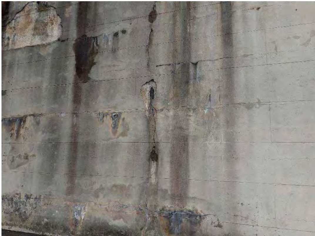
Figure 8: Cracks in the render at the location of SBR 3.3 (prior to the installation of the protective mesh).
