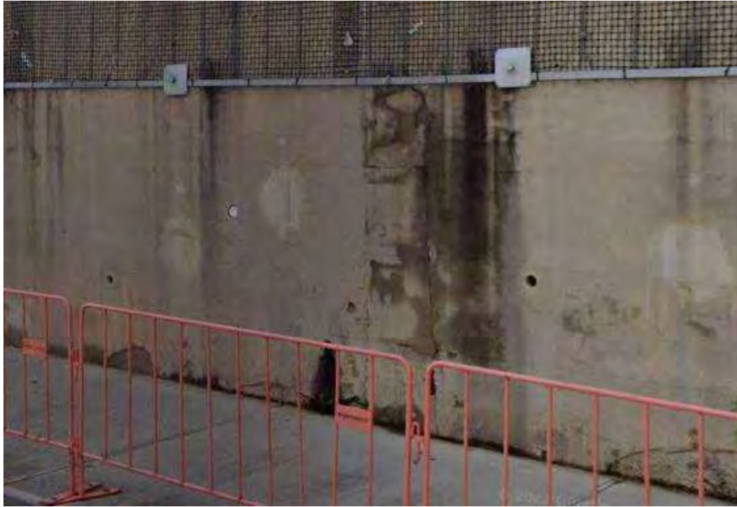
Figure 7: Cracking at the location of SBR 3.2.
