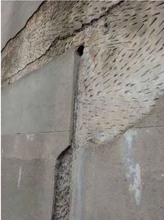
Figure 13: Exposed patches of render indicate that at least some sections have three layers of render and the lower layers are pecked to create a rough surface for the next layer.
