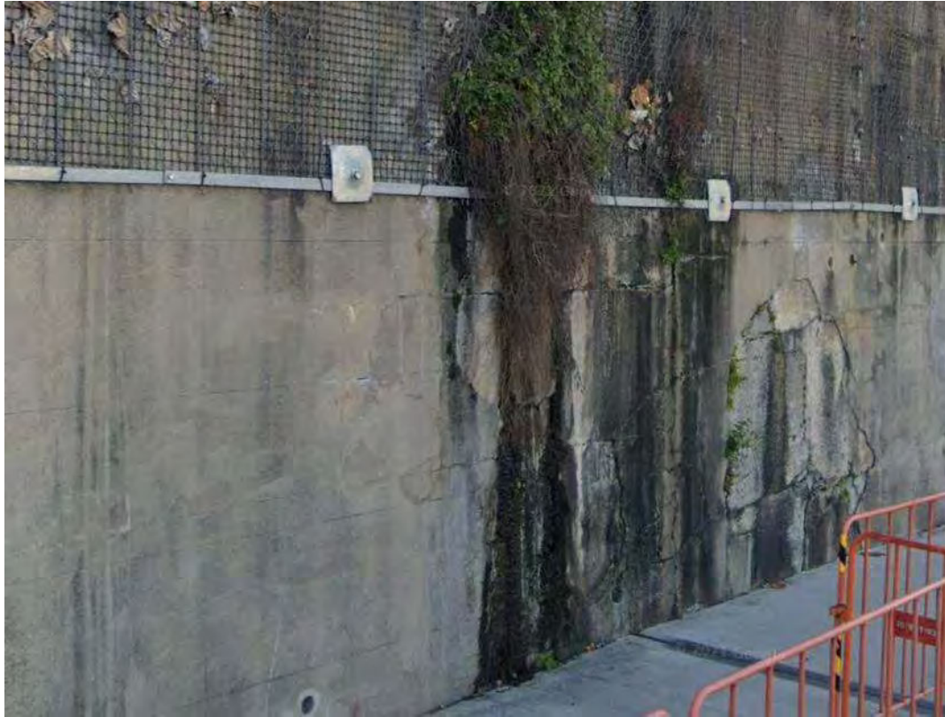
Figure 9: Cracking and intrusive vegetation at the location of SBR 3.4.
